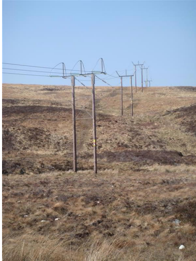
Photo 3.1: Illustrative image of temporary wood pole.
