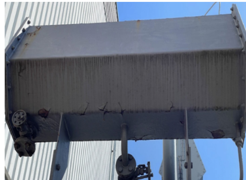
Earthing Transformer Corrosion
