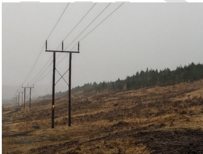
Plate 2.1. 'H' Trident Wood Poles
