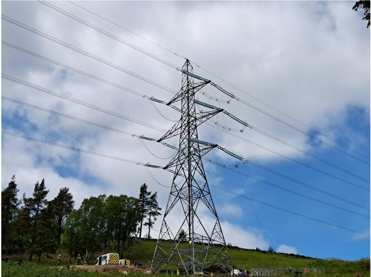
Photograph 3-1 Tower showing twin conductor on left and triple conductor on right
