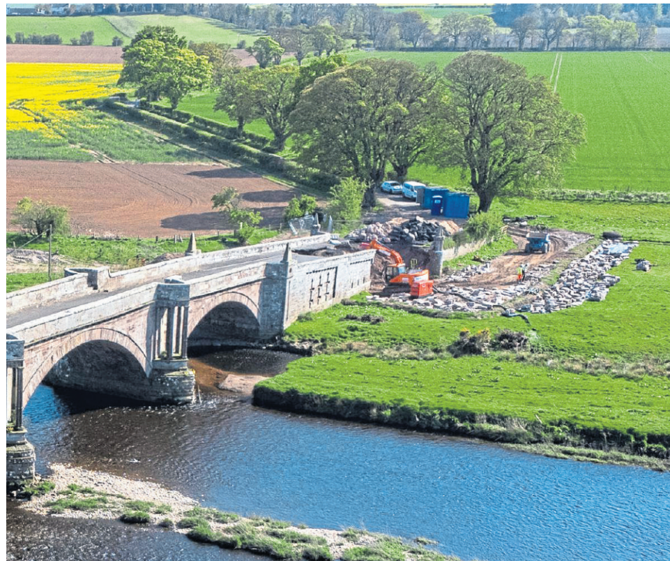
AERIAL VIEW: Drone footage of the repair work being carried out at Bridge of Dun, near Montrose, after it was damaged during Storm Babet. Picture by Kim Cessford.
