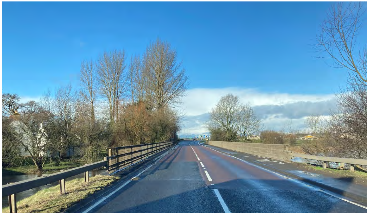
3a. Continue on A84 for 0.3 mile. Cross River Forth Bridge – to be checked by BEAR Scotland.
