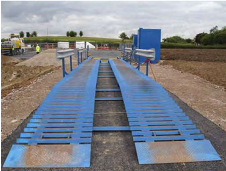
Plate 3.13: Vehicle wheel wash facility
