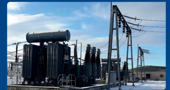
Existing transformers to be replaced
