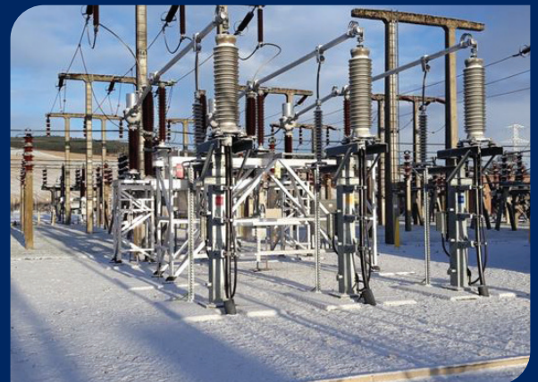
Ageing 132kV equipment required to be replaced.
