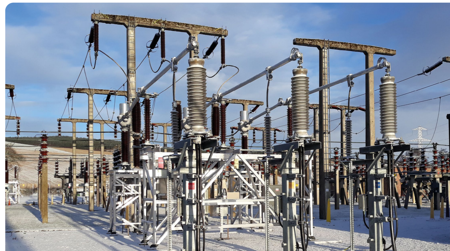
Existing AIS equipment required to be replaced
