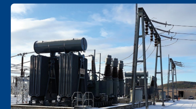
Existing transformers to be replaced
