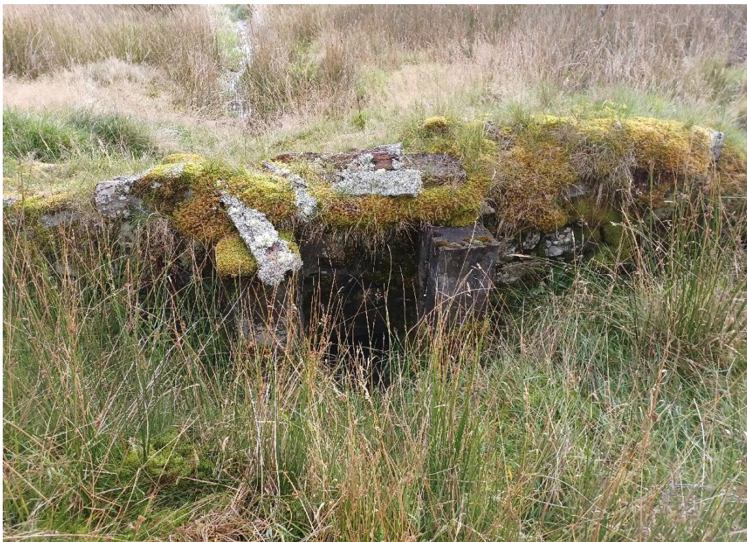
Plate 6.2 - Lade dam approximately 5m over a lade extending from Johnstripe farmstead to the south. Identified during walkover survey on October 21, 2021.
