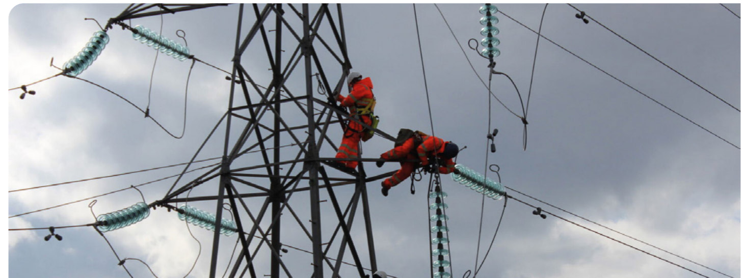
The above image shows the construction of a new steel lattice tower.
