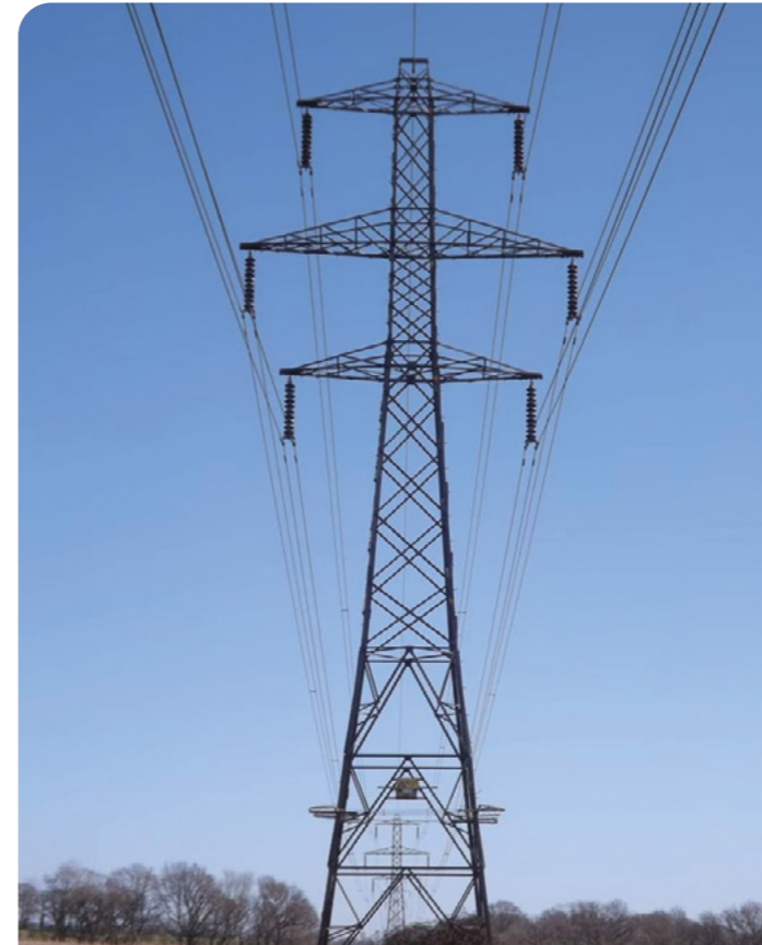
A picture of an operational steel lattice tower, similar to the technology being proposed for this project.
