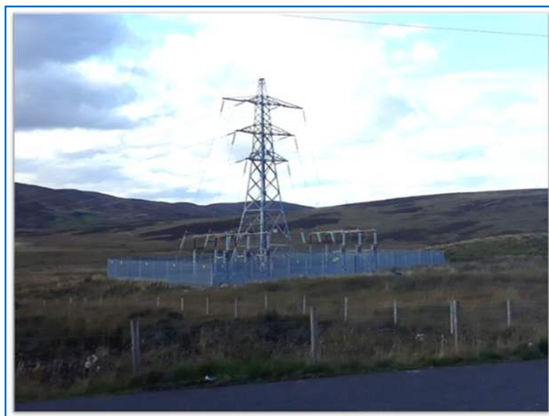
Plate 3.4: Example of a Cable Sealing End Compound
