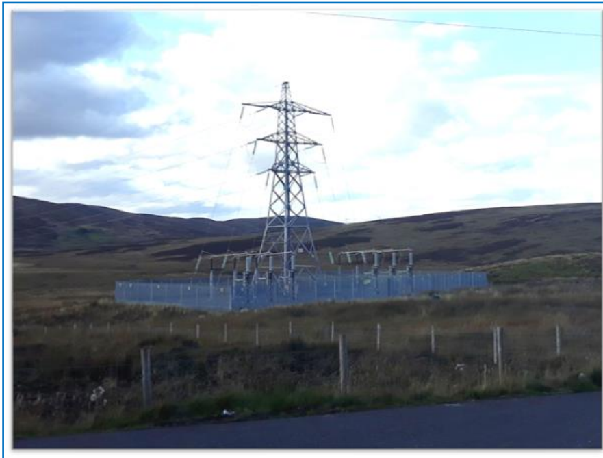
Plate 3.6: Example of a Cable Sealing End Compound
