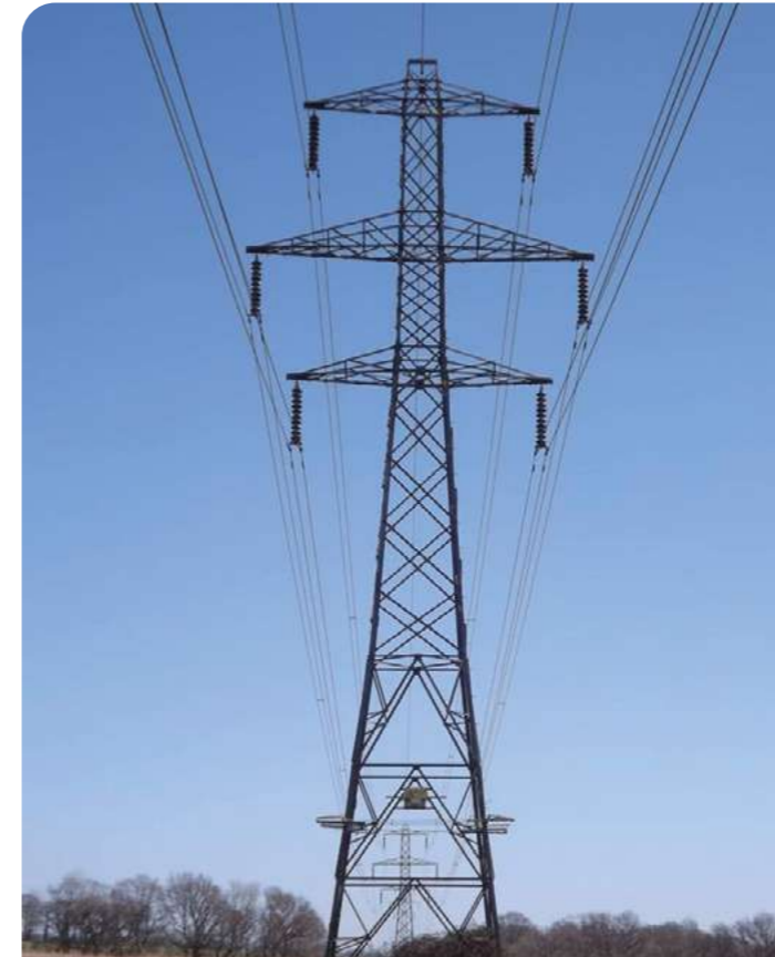
A picture of an operational steel lattice tower, similar to the technology being proposed for this project.
