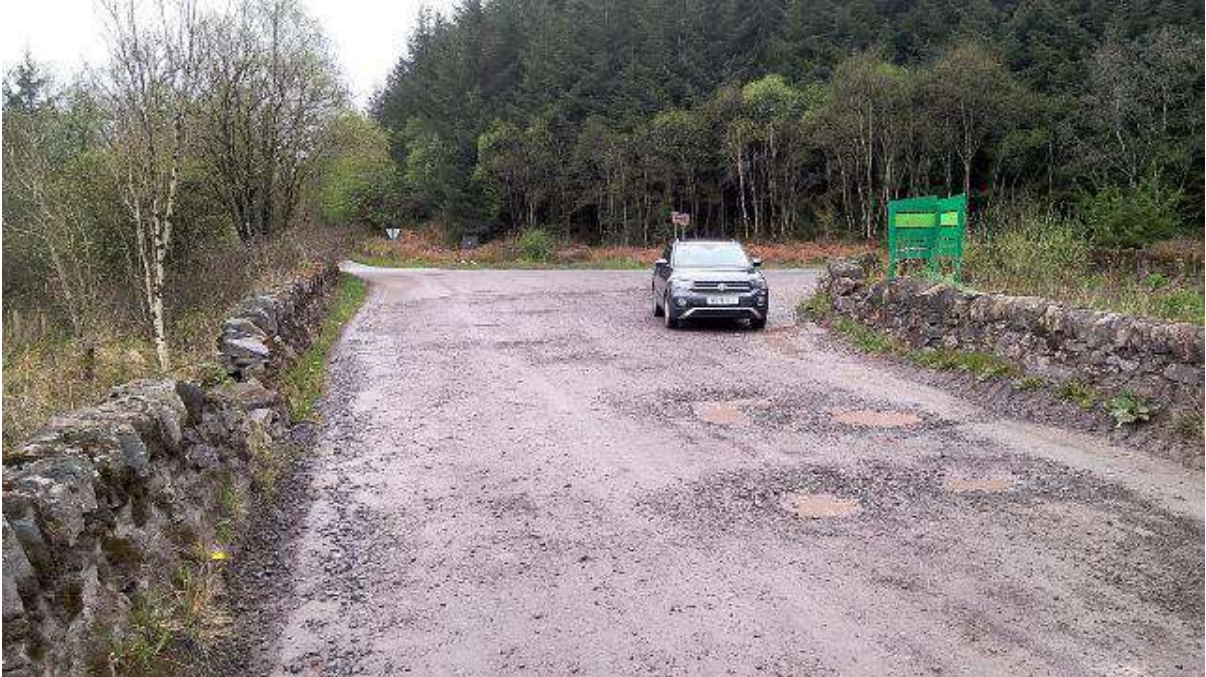
Plate 11 – A view of the bellmouth of the existing access road looking out onto the A816.
