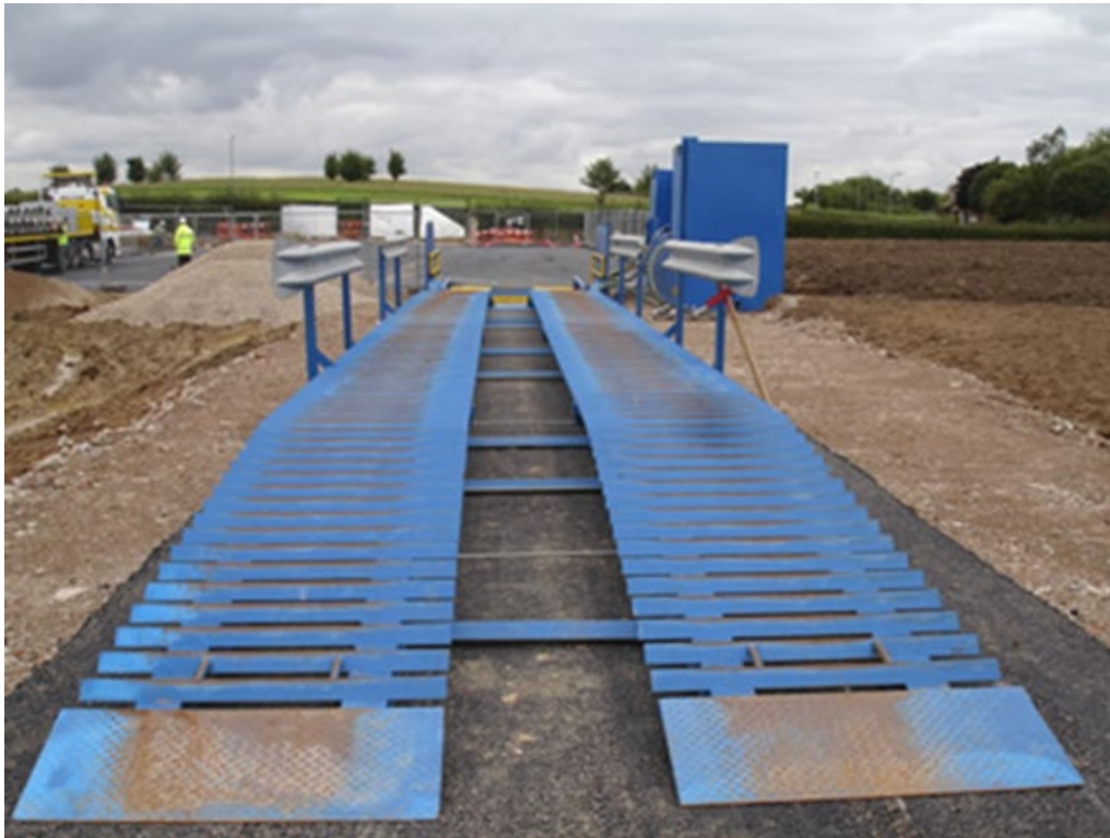
Plate 3.12: Vehicle wheel wash facility
