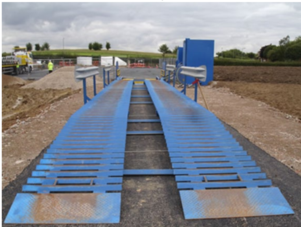
Plate 3.12: Vehicle wheel wash facility
