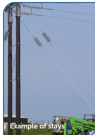
Typical single circuit double trident wood pole
