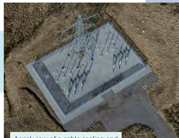
Aerial view of a cable sealing end
