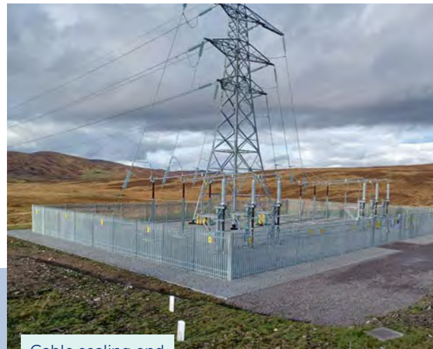
Cable sealing end
