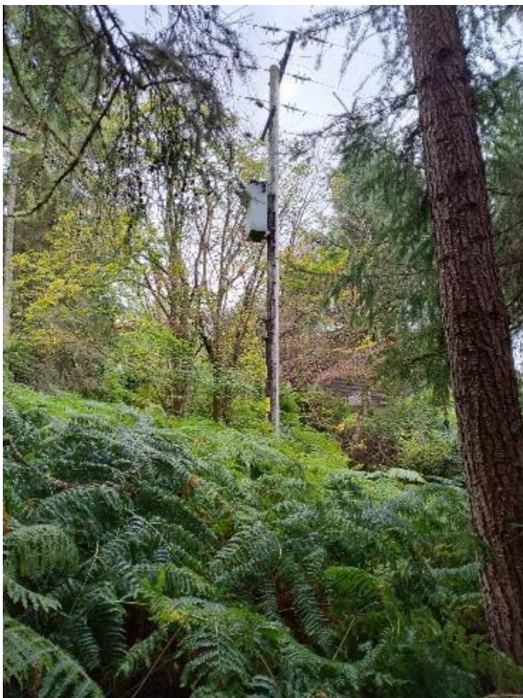
Plate 15: Distribution overhead powerline
