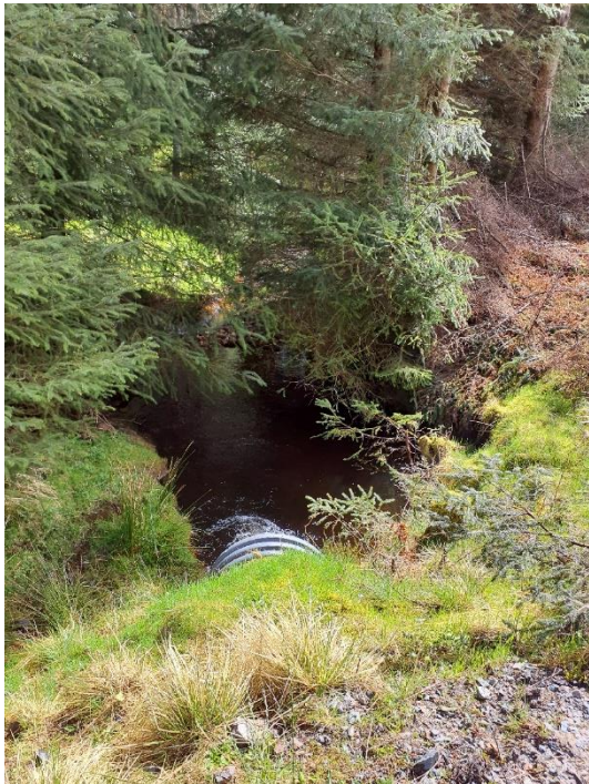
Photo 7: Example of the typical pipe culverts and watercourses present within the Site
