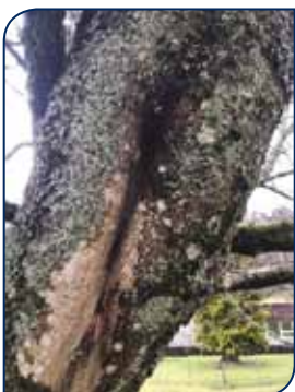
Two crack features with bat roost potential on trunk of an Acer platanoides (Norway maple) within Site 3.
