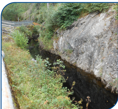
Engineered canal which is part of the Lochay power station operations.
