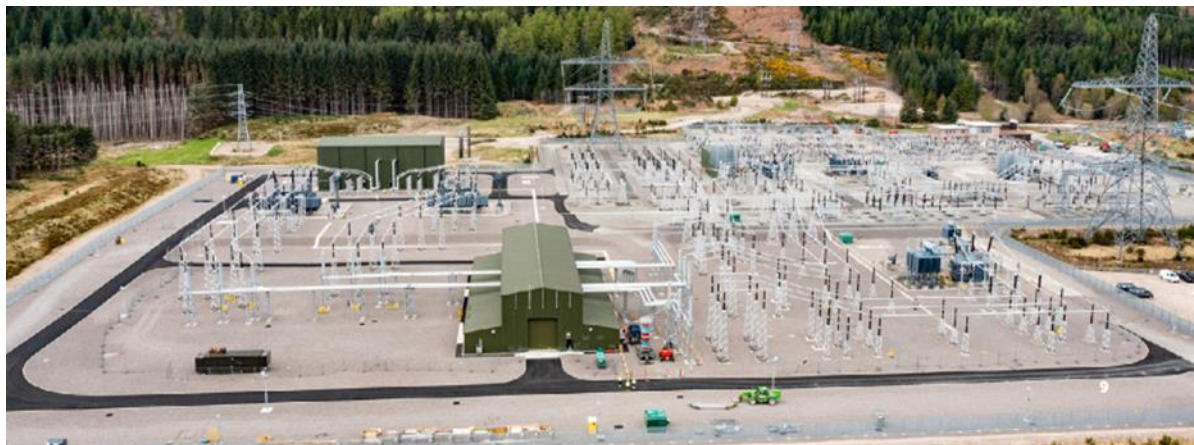
Plate 3-1 Example 400 kV Substation
