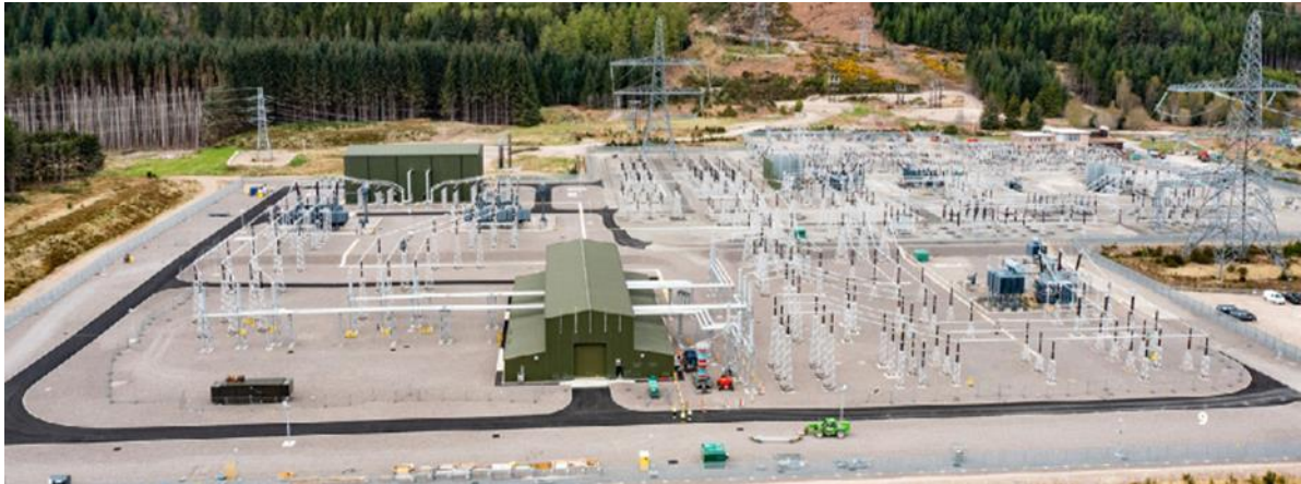
Plate 3-1 Example 400 kV Substation
