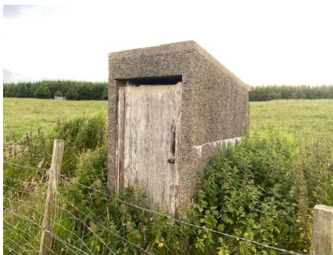
Figure 9.7.4 Private Water Supply (PWS) access point
