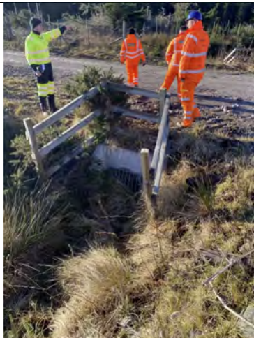
Photo 2.12: Substation surface water culverted under access track
