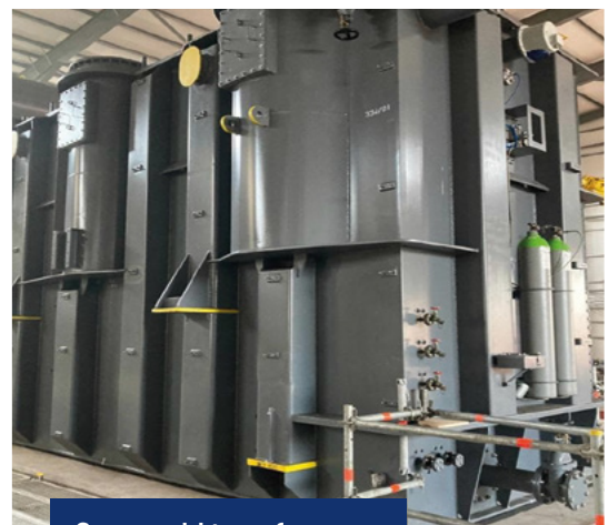
Super grid transformer
