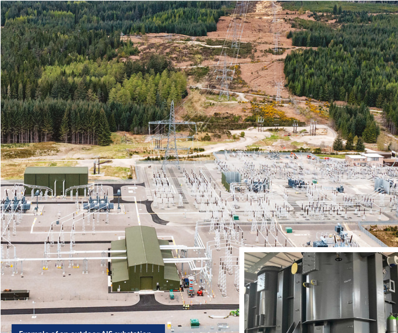
Example of an outdoor AIS substation
