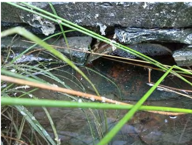
Photo 2.3 250mm Steel Pipe Outlet
