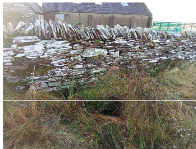
Photo 4.6 150mm Stone/Concrete Pipe. 50% Blocked.
