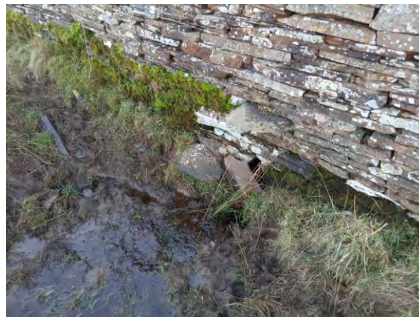
Photo 3.9 Masonry/stone box built into wall. 250mm wide, 600mm high.
