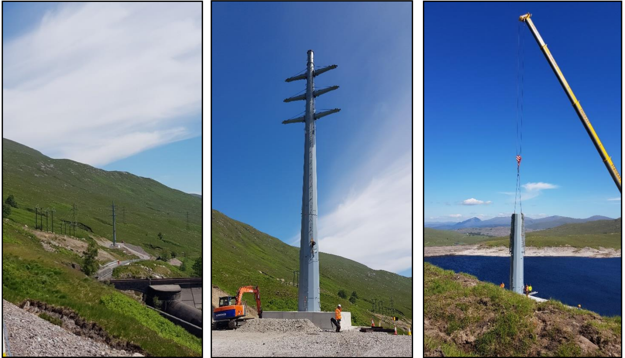
Plate 7.1: Example of NeSTS pole with larger 400m+ spans
