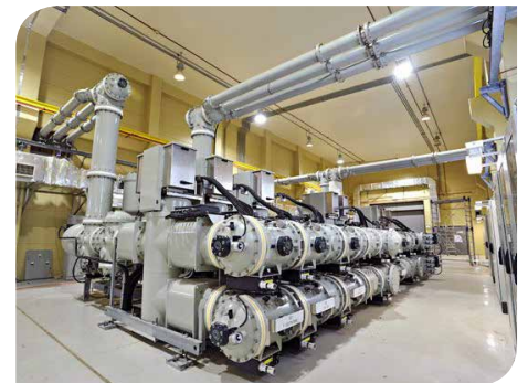
Inside of a GIS substation
