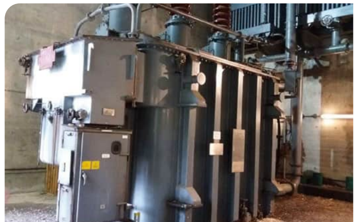
Existing internal transformers needing to be replaced (at Aigas & Kilmorack)
