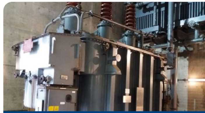
Existing internal transformers needing to be replaced (at Aigas & Kilmorack)
