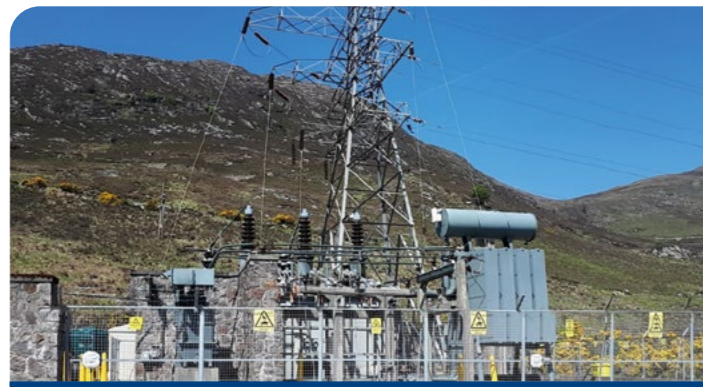
Existing external transformer arrangement needing to be replaced (at Deanie & Culligran)
