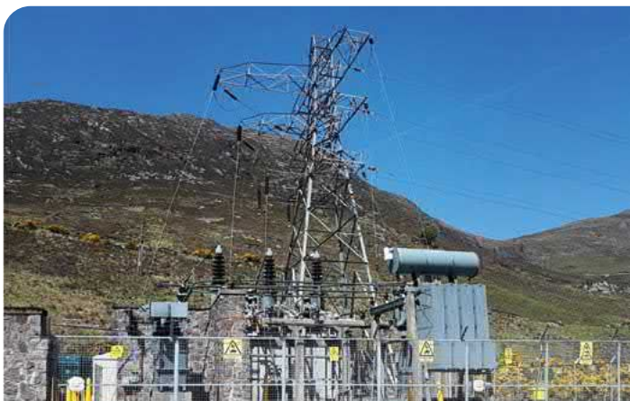
Existing external transformer arrangement needing to be replaced (at Deanie & Culligran)
